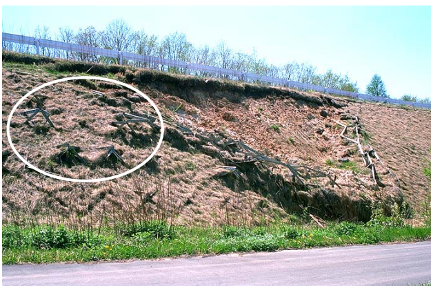
Figure 1. Surface failure on the artificial slope and frost heave damage to protective grids, marked with a circle (left).
